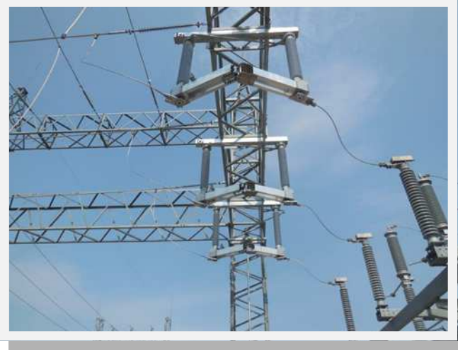
Kashechewan TS: new disconnect switch for transformer
