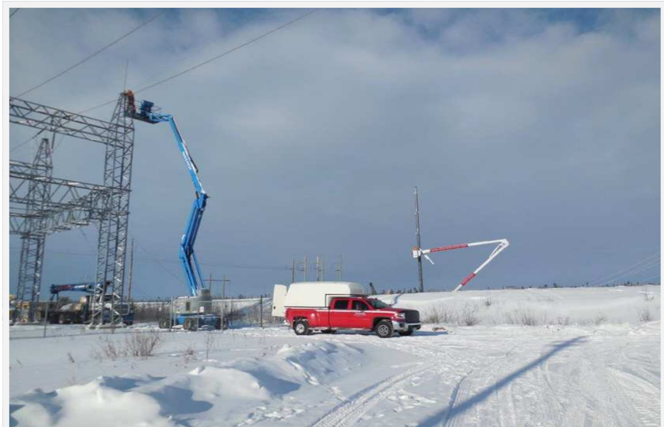
Kashechewan bypass link, behind the berm wall, installed in March 2016
