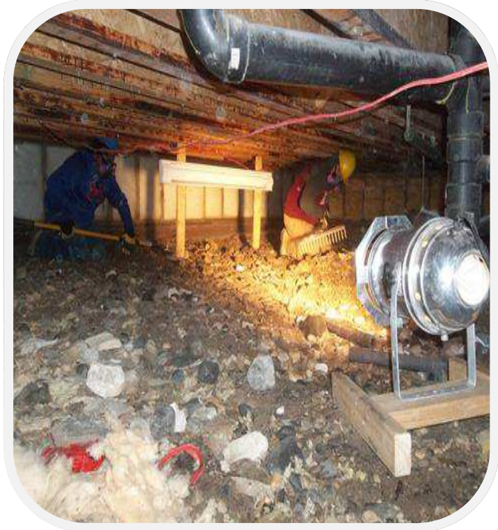
CotC crew preparing the earthen crawlspace to be covered by a moisture barrier.
