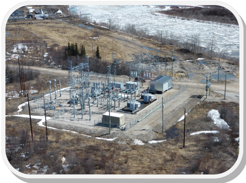
FNEI Substation in Attawapiskat.
