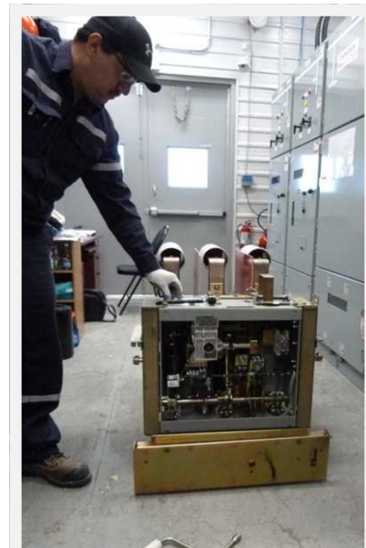
Above: Mr. Tony Iserhoff doing testing & maintenance at one of our substations.
