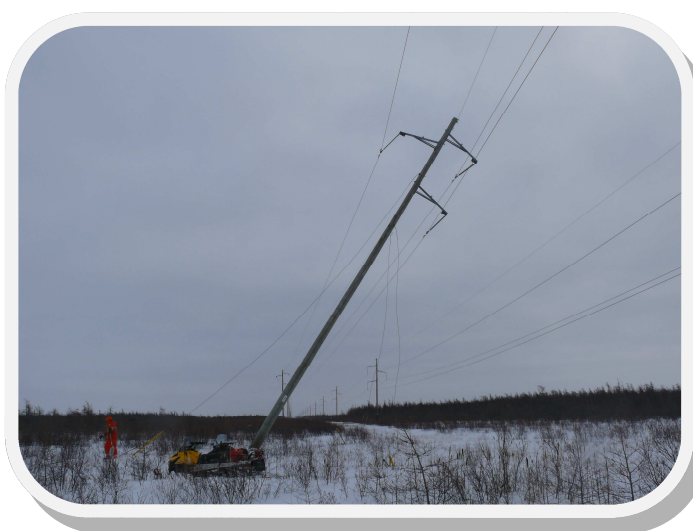
Pole Repair: a new pole is being put up and is no easy task-care, safety, for all involved, is at the forefront when doing this work!
