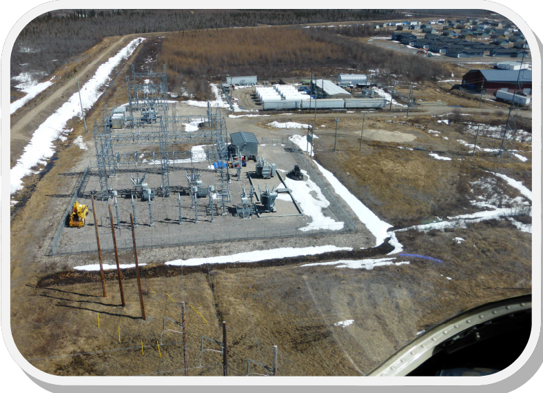
FNEI Substation in Kashechewan.
