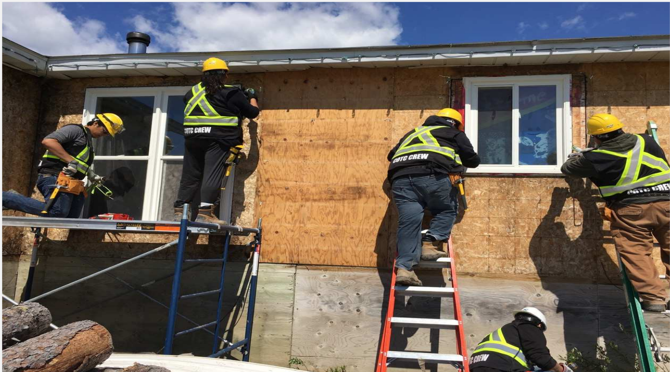
Above: The Conservation on the Coast Kashechewan crew busy retrofitting a home in Kashechewan!
