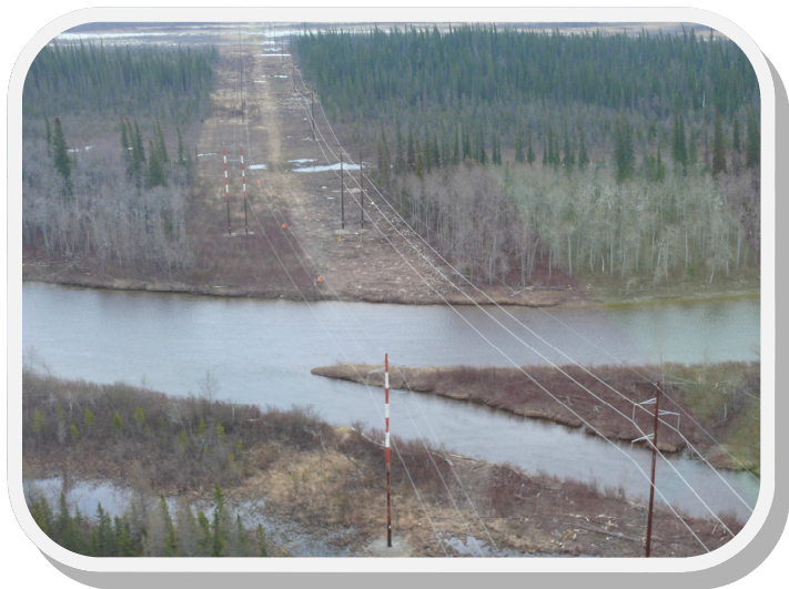
FNEI Transmission Line crossing a river.
