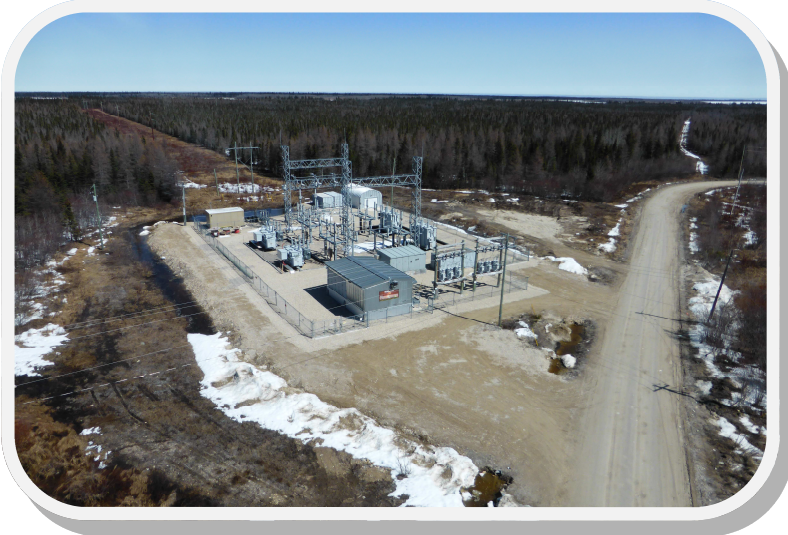
FNEI Substation in Fort Albany.
