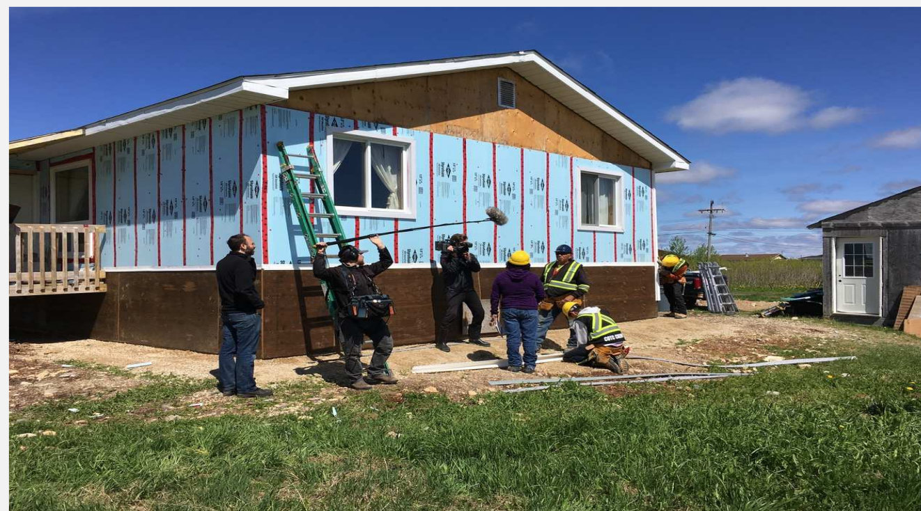
Above: Video Filming in June 2017, in Fort Albany, of the Conservation on the Coast Fort Albany crew in action-they are busy retrofitting a home.
