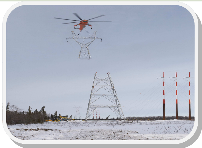
Special helicopter used to place top part of tower to bottom half of tower.
