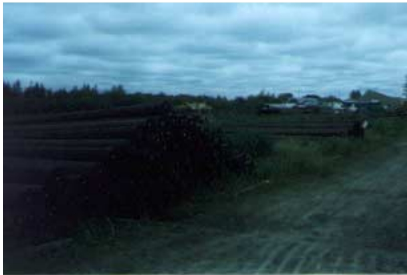
These are only a few of the over 1600 poles that will be used in the construction of the Omushkego Ishkotayo transmission line. Pole lengths range from 75 feet to over 100 feet long and are treated to resist rot and insects for a minimum of 40 years.
